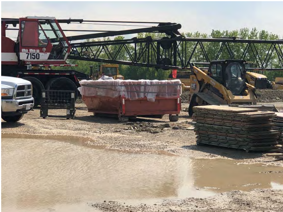
Figure 2: Concrete washout bin is on stable ground and no leakages were observed; view to southwest.
