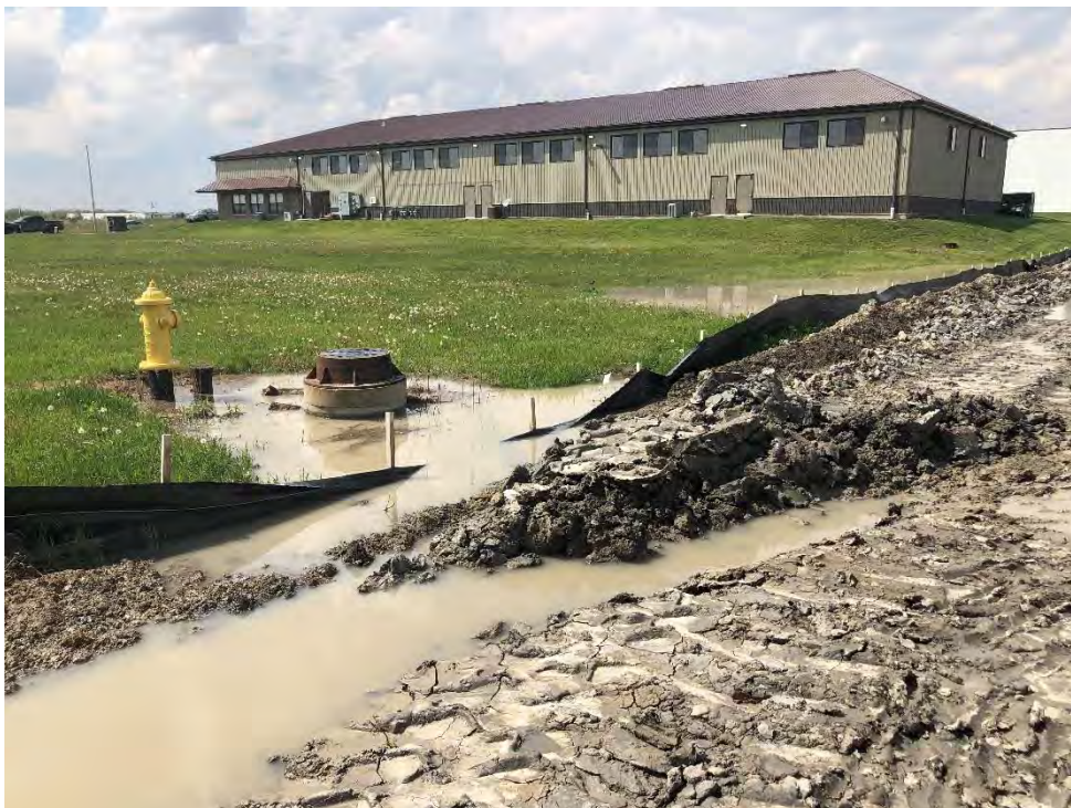
Figure 4: Silt fence along the southwestern perimeter has been blown off the stakes and is allowing stormwater off-site; view to northwest.
