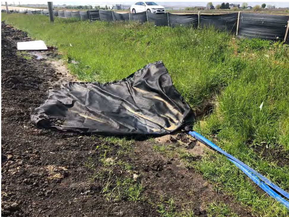
Figure 8: The storm drains are being dewatered through a filter bag along in the northeast corner of the site; view to northwest.
