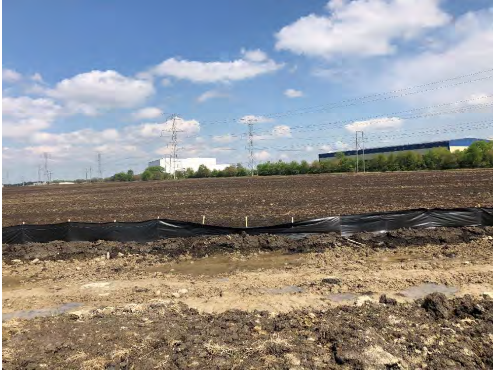
Figure 1: Silt fence has blown off the stakes in the construction area east of McLinden Road; view to east.
