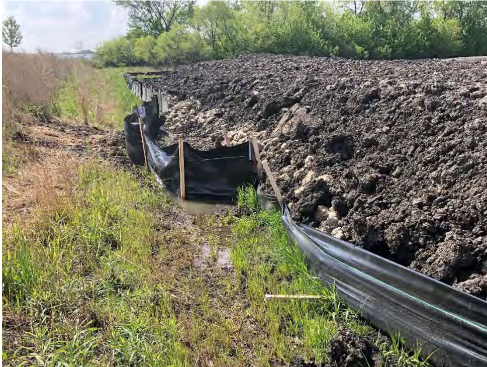
Figure 5: Newly installed silt fence along the southern perimeter has not been installed properly and is allowing stormwater to undermine the silt fence; view to west.
