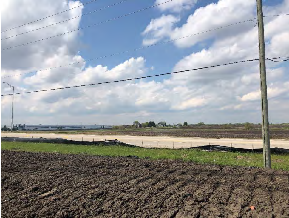
Figure 3: Silt fence has blown off the stakes along the northern perimeter of the site; view to north.
