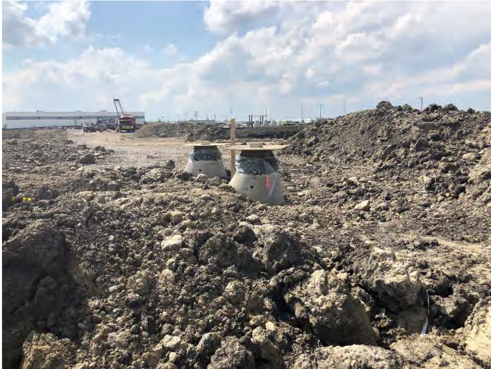
Figure 7: Storm drains are currently above grade. Grates and inlet protection baskets should be installed as soon as possible; view to northwest.
