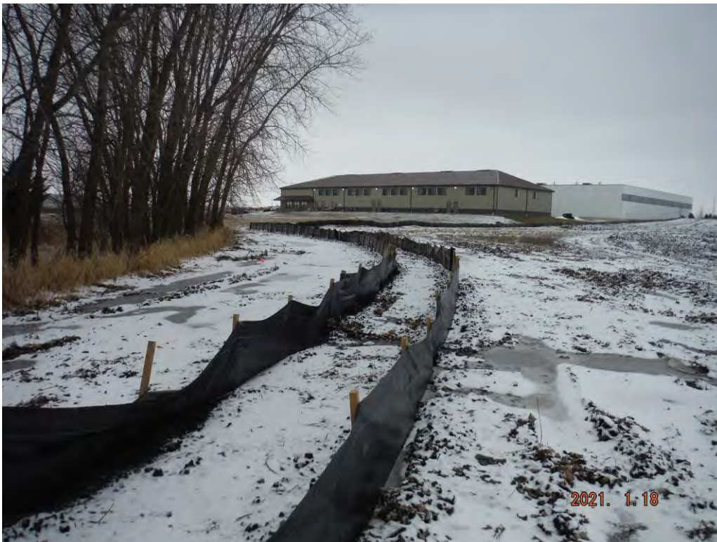
Figure 4: Double silt fence in good condition along southwest perimeter of Site and adjacent to wetland; view to northwest.
