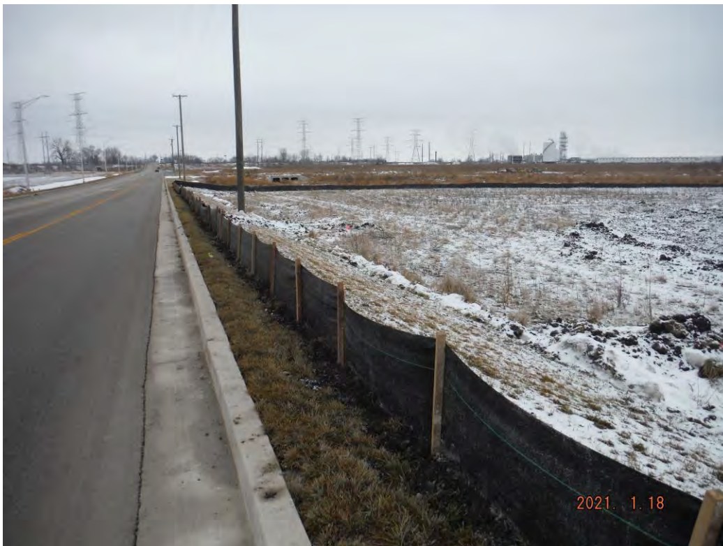
Figure 6: Silt fence in good condition along east perimeter of Site; view to south.
