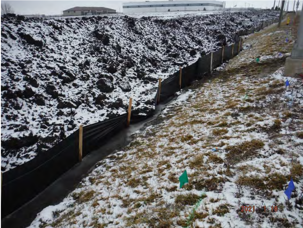
Figure 1: Silt fence damaged by mass grading along north perimeter of Site; view to west.
